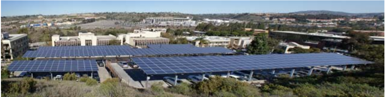
The solar carports at the District offices are among several carport installations throughout the District, part of a 20-year Power Purchase Agreement with Borrego Solar.
